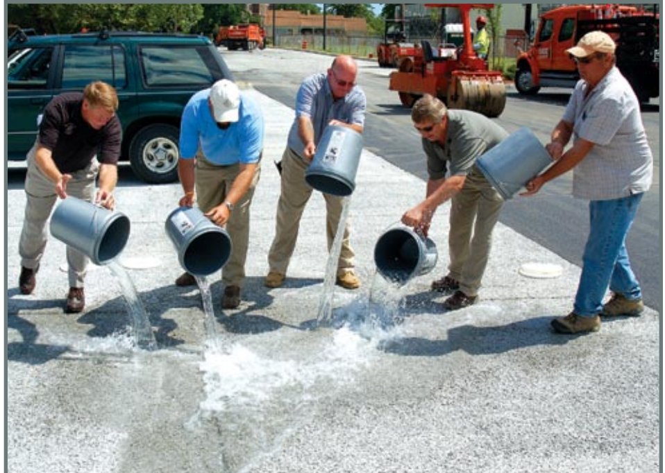
From left to right: Stephen Martin, P.E., City Engineer, City of Williamsburg, Phil Sabo, General Manager of Branscome, Andy Mckown, General Superintendent of David Nice General Contractor, Jack Kowalski, Quality Control Manager of Branscome, and Rick Hite, Concrete Contractor for Rick Hite Concrete.
