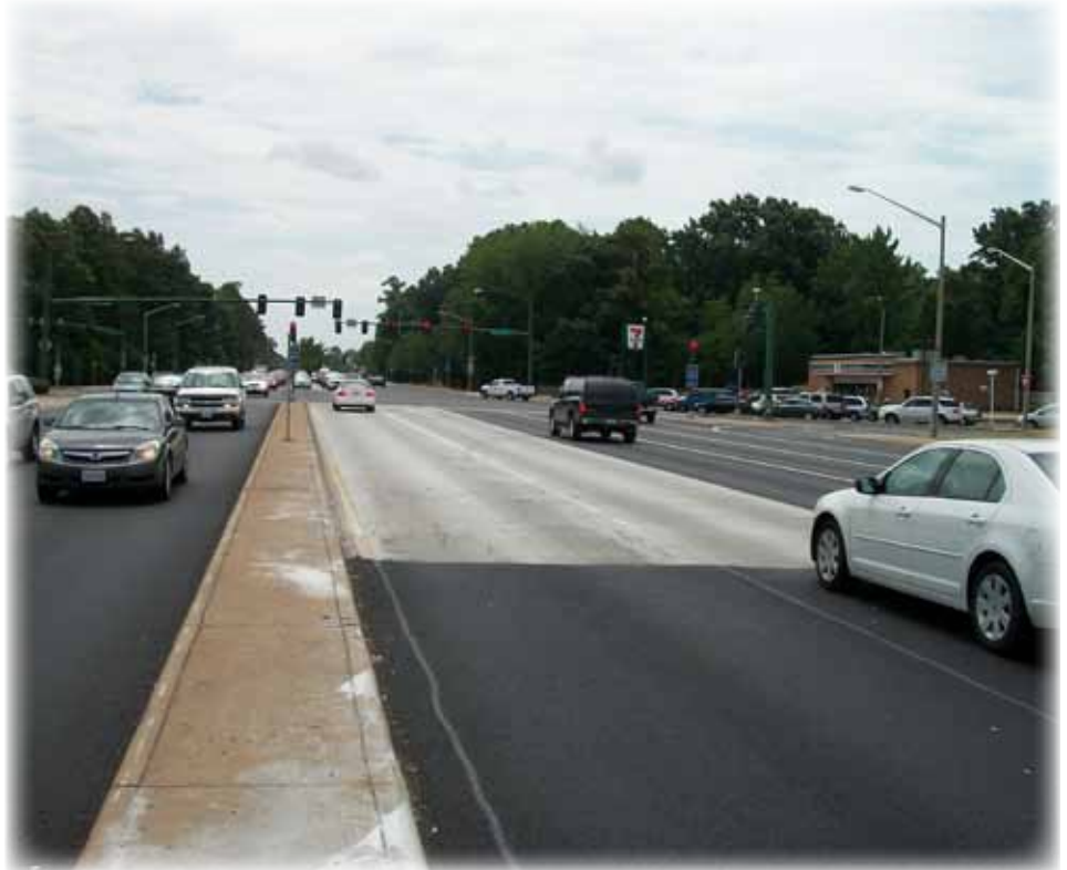
Newport News concrete turning lane—part of the VRMCA local streets and local roads program.
