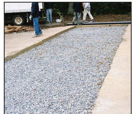
Six inch rock storage bed.
