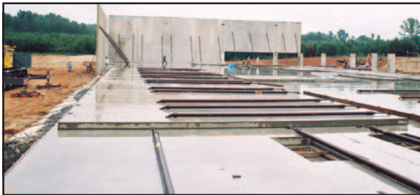
The Tilt-up process of a north section being erected, with panels waiting for lift up.
